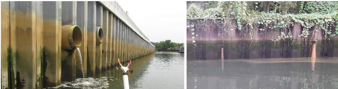
Discharges from outfalls along Glen Cove Creek at north bulkhead (l) and south bulkhead (r) (photos by Carol DiPaolo, 6/2/21 and 9/22/21, respectively)
