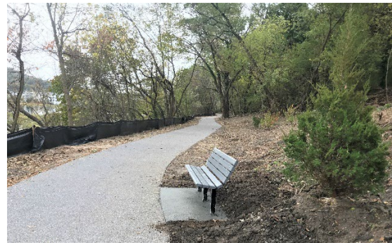
Starting point of the Hempstead Harbor shoreline trail and extension south along the western shoreline (above l and r) (photos by Carol DiPaolo, 5/20/15 and 9/16/20, respectively); the trail was completed and new plantings installed by the Town of North Hempstead in 2019 (r) (photo by Kevin Braun, 10/22/19)
